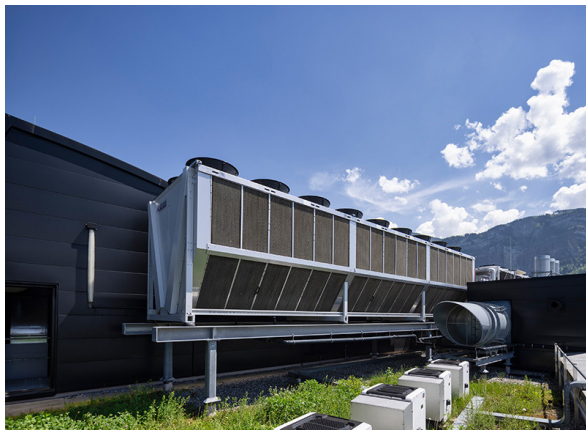
Pictures: New chiller with free cooling and recooling on the roof
