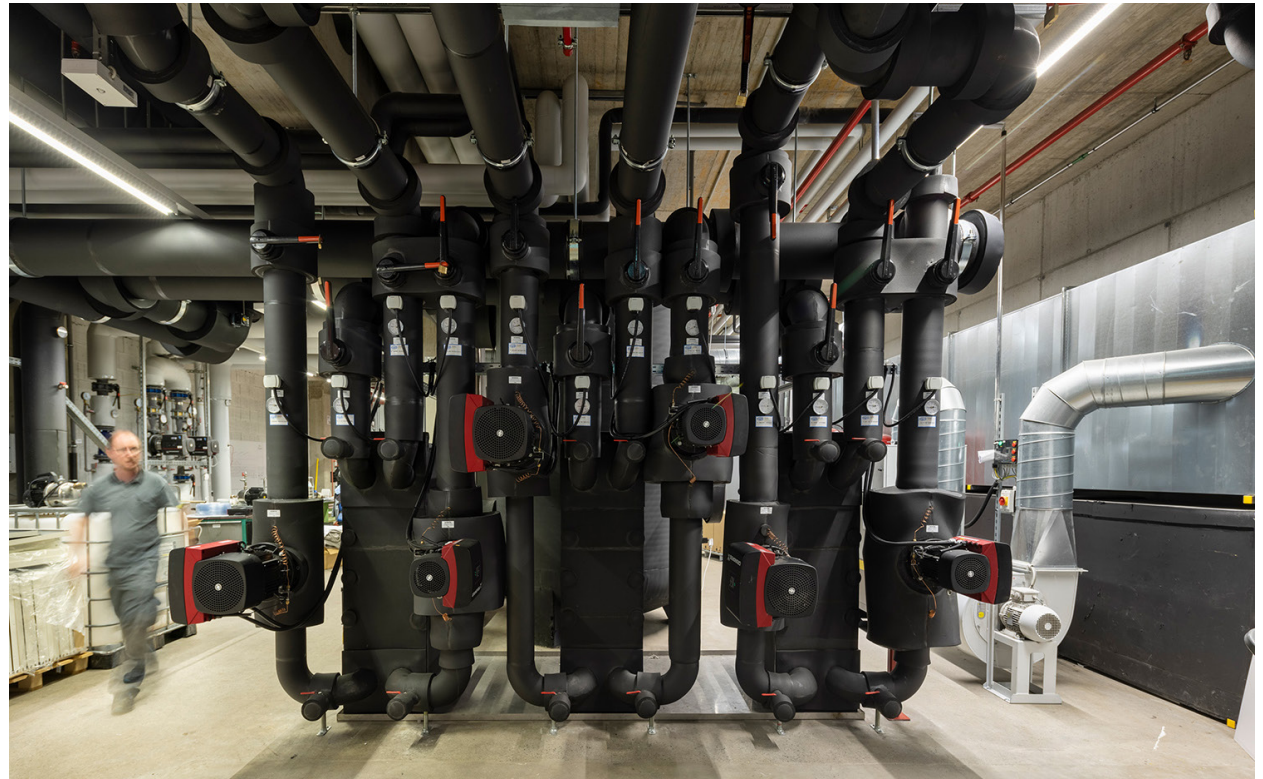
Picture: New refrigeration supply centre at the Dornbirn Schweizerstraße
